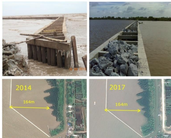
Figure 2-4 Typical location where the CB was installed at Khanh Tien Commune, U Minh district, Ca Mau Province (Location 4), and pictures in 2014 and 2017 indicated poor natural mangrove tree development
