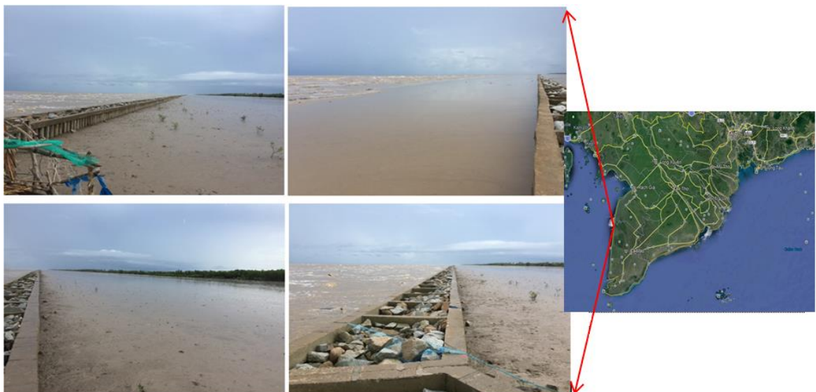
Figure 2-5 Some pictures of the existing situation of the first type of CBs at Ca Mau in July, 2017.
