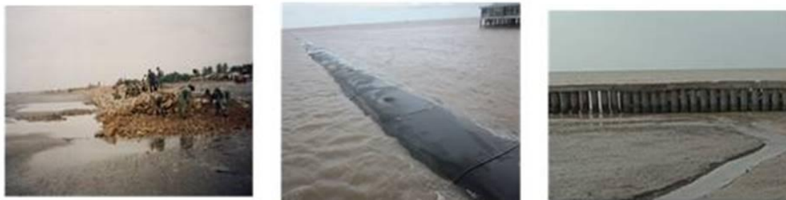
Figure 4. Breakwater by riprap (G2- Can Gio), geotube (G3- Bac Lieu), and concrete piles (G1- Ca Mau)
